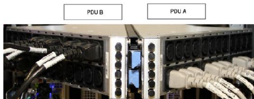
Figure 11 Power distribution unit (PDU) without installed wire bales, rear view
